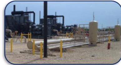
LMS Gas Lift Compressor Station
