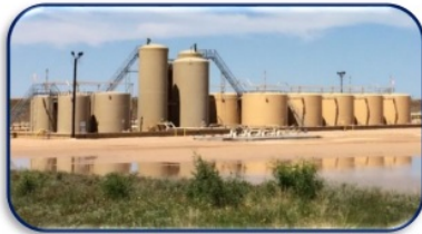
LMS Water Treatment Plant
