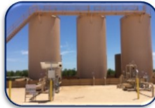
LMS Crude Gathering Tanks at Reagan Truck Station
