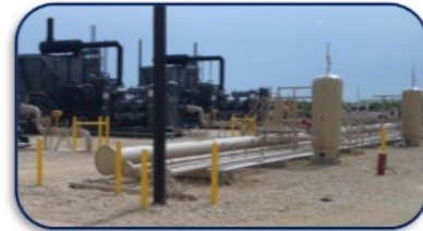
LMS Gas Lift Compressor Station
