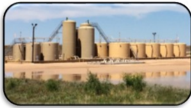
LMS Water Treatment Plant
