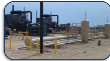
LMS Gas Lift Compressor Station
