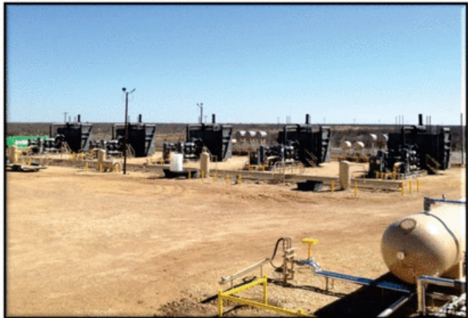
Reagan North Centralized Compressor Facility
